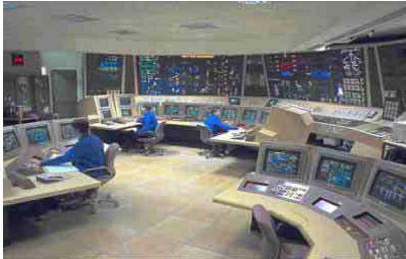
N4 Control Room
