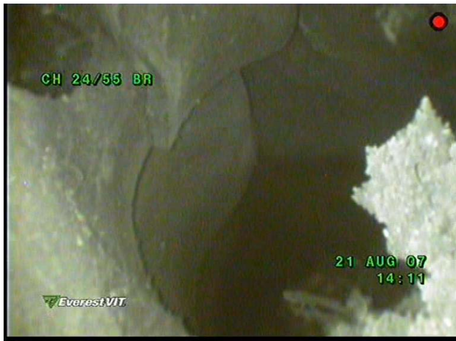
Figure II—Graphite Damage/Displacement In A Fuel Channel.
