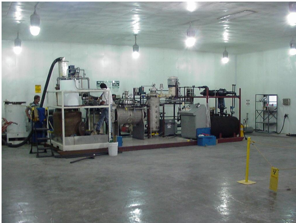
Fig. 6. Complete SL-2 SET Plant, capable of treating 500 lbs/day of diverse waste types
