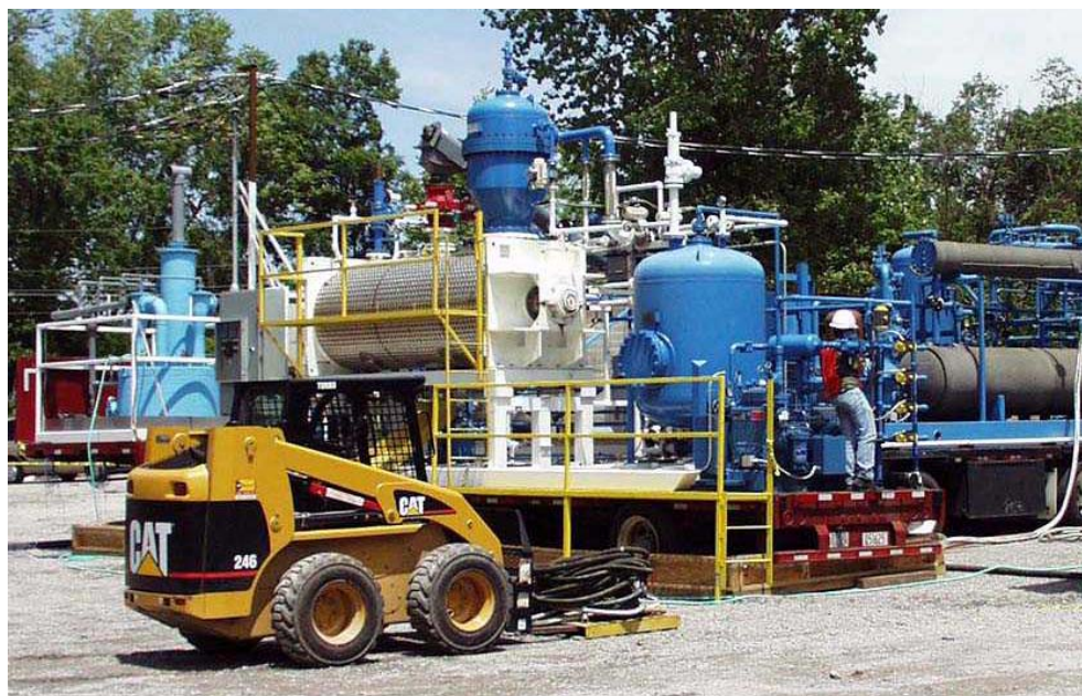
Fig. 1. SET™ S-10 in Operation
