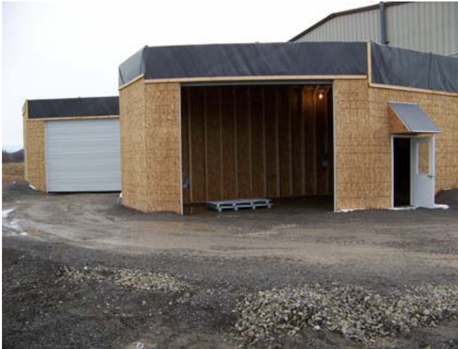
Fig. 5. The construction of two temporary weather shelters provided additional working space for package finalization and tagging.
