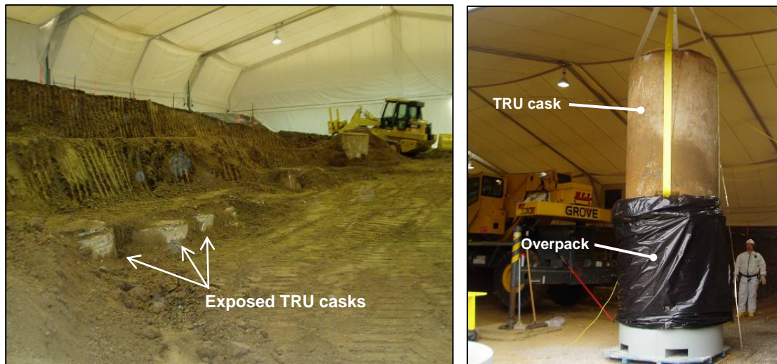
Fig. 3. Excavation showing exposed TRU casks ( left ) and the transfer of casks to overpack ( right )
