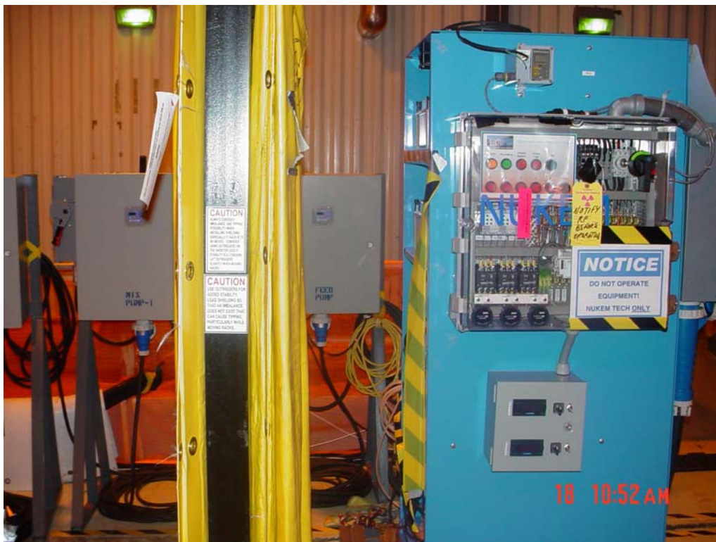
Figure 5. EC Control Panel and Chem-Feed and Grinder Pump VFD Panels
