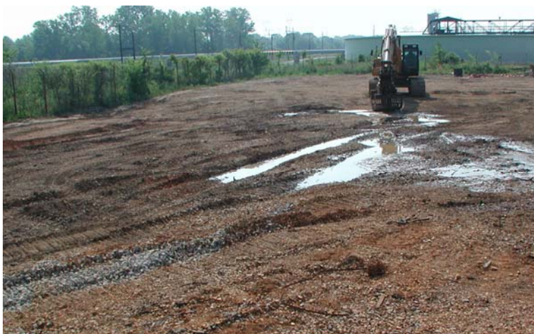
Figure 3. A view of the LRA after removing the deteriorated drums and lead turnings.
