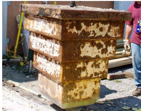
Fig. 9. Steel jacketed concrete plug from the hot pipe tunnel prior to remediation efforts.
