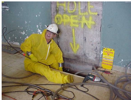
Fig. 16. BSI worker feeds combination of camera and abrasive tool into conduit, while watching his progress on a television monitor.
