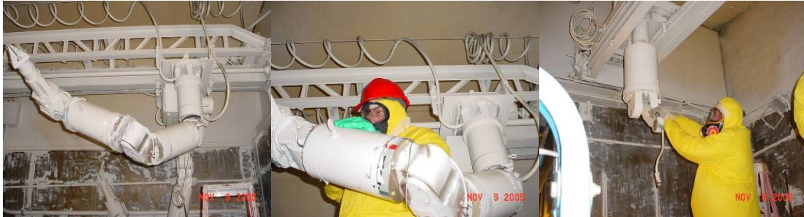
Figs. 4, 5, 6. – Worker removing manipulator arm – note arm is coated with lockdown to control loose contamination. Also note the hot cell stainless steel liner visible in the background. (Hardhat requirements in the cell were waived by the time work progressed to the point of Fig. 6).
