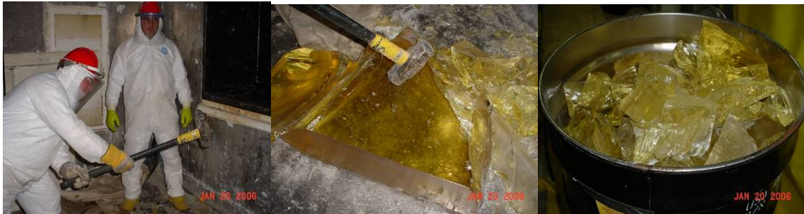
Figs. 9, 10, 11. Workers size reducing hot cell leaded window slabs, shards disposed of in drums. The glass slabs often cracked as they were being slid carefully out of the frame, due to their extreme brittleness. Size reduction was very quick work.
