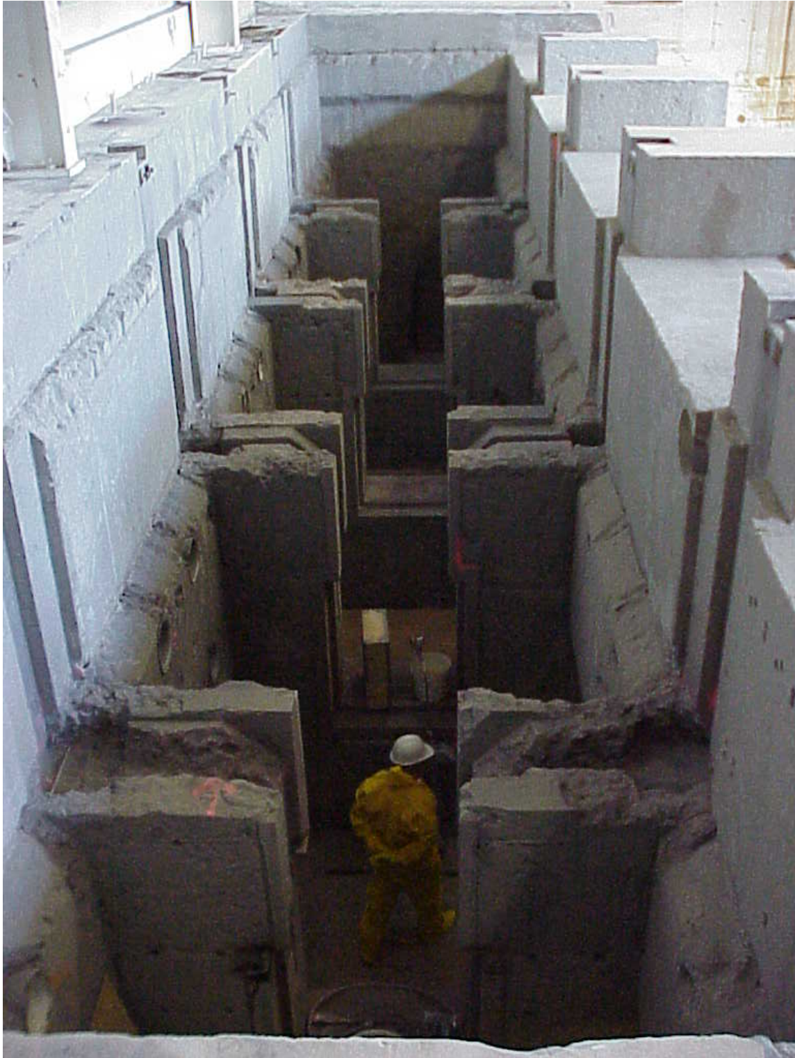
Fig. 18. The view looking down into Hot Cells #3 - #7 with the roof slabs and transfer doors removed, and decontamination to the Remedial Action Limit (50% of the DCGL) complete. This area is ready for Final Status Survey.
