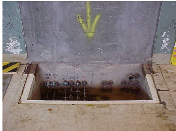
Fig. 15. Access hole to conduit in hot cell, located in the front wall of the hot cell directly beneath the former manipulator operator position. Ends of the conduit are plugged for isolation control when cleaning is not in progress.
