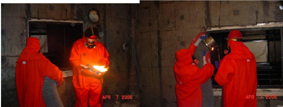
Fig. 12, 13. Workers cut out the steel window frames after removing all lead shielding, including lead impregnated wool, lead bars, and lead shot.
