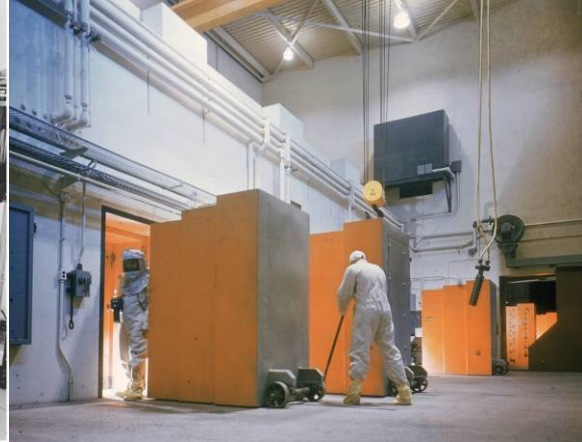
Fig. 2. Rear of hot cells
