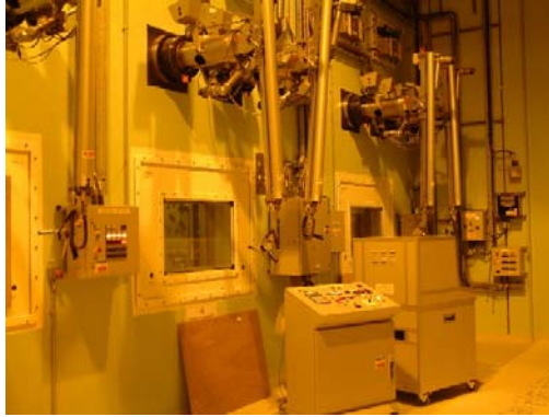
Figure 3 One of the highly active cells in the Technology Centre
