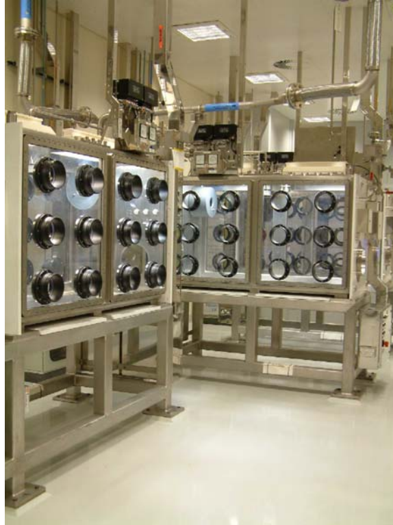
Figure 2 Part of the Alpha-active Facilities in the NNL's Technology Centre
