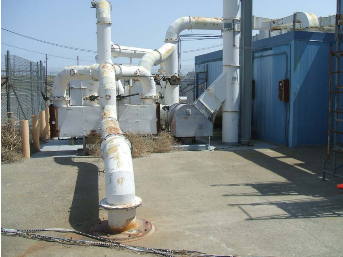
Figure 3. Original Deactivated HVAC System
