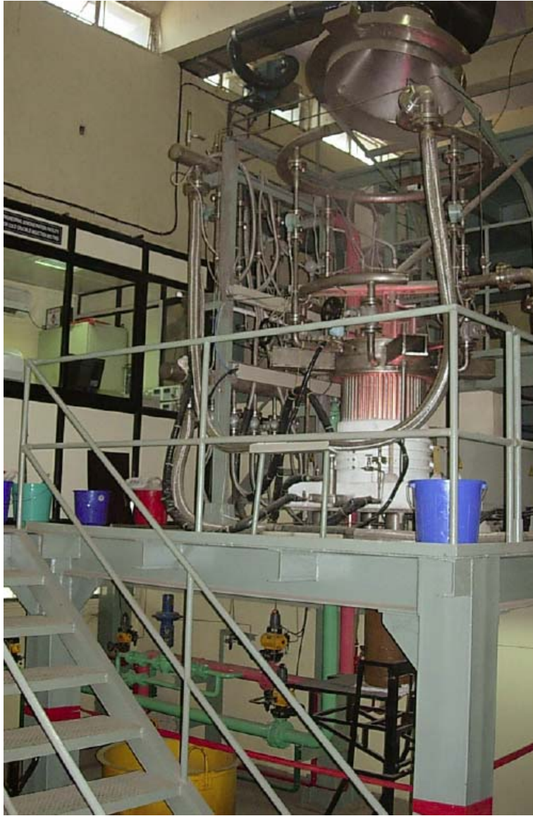
Fig. 2 Engineering scale facility for cold crucible induction melting
