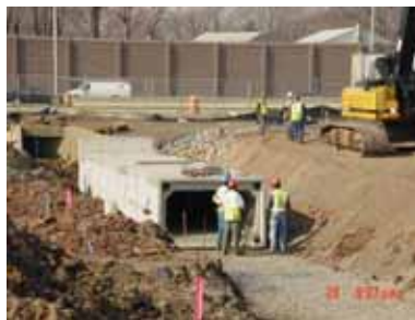
Fig. 3. Installation of new pre-cast concrete culvert sections at the 160/174 Essex Street property.
