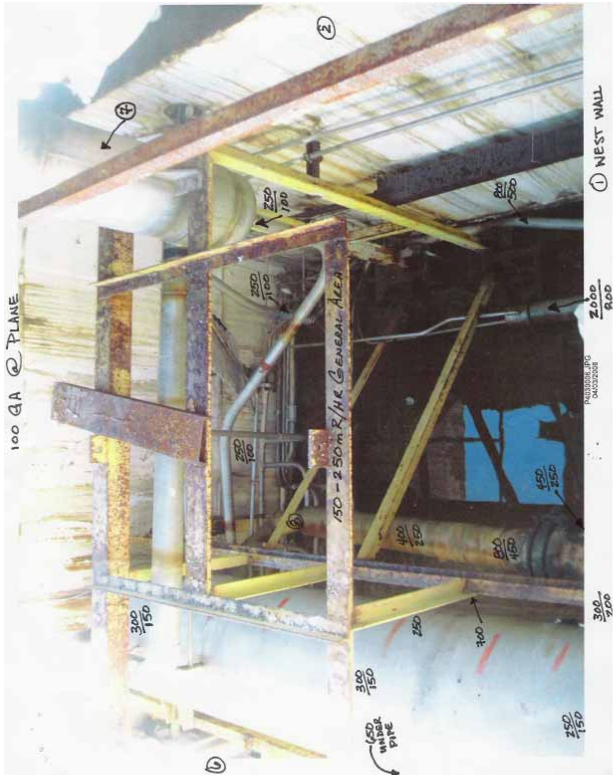
Fig. 3. 7502 Waste evaporator and associated piping with measured doses (Surface/30cm).
