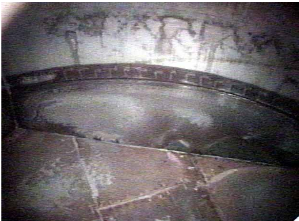
Fig. 3. TFF Tank WM-186 post-decontamination interior.
