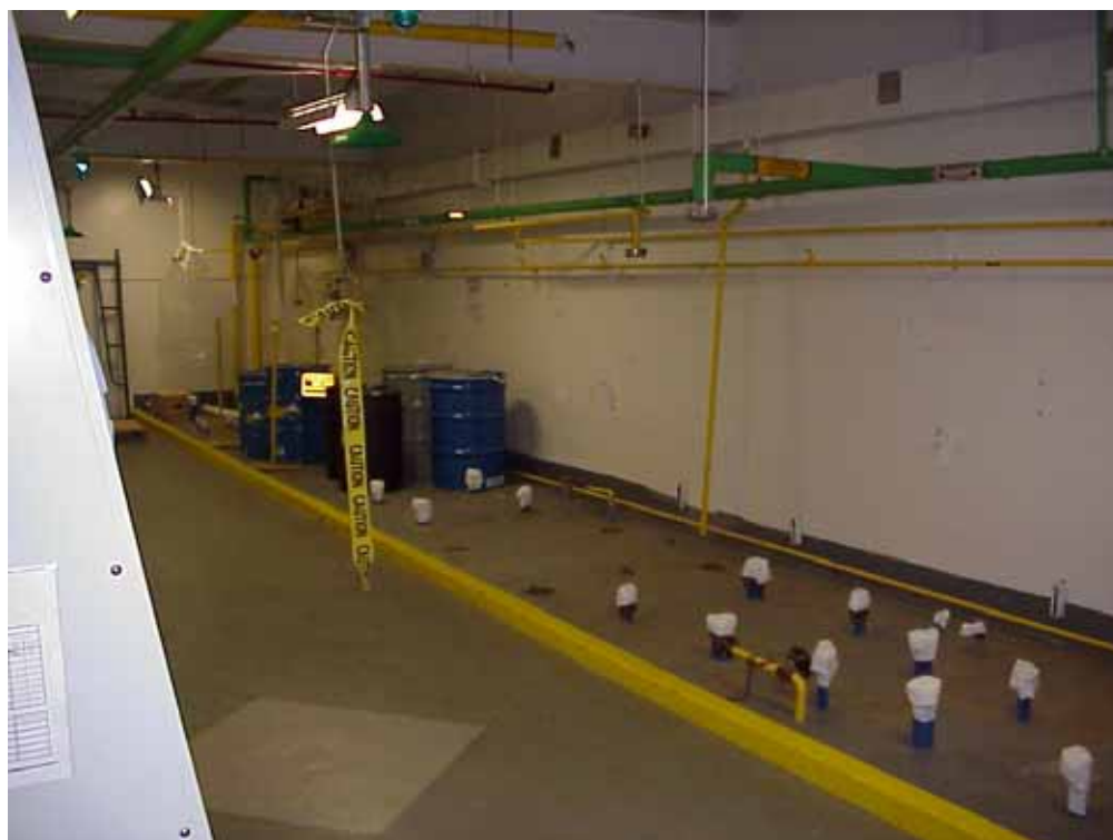
Figure 1 – The removal of the bulk chemical feed tanks and draining of the chemical feed lines from rooms 336 and 337 is one of the many efforts to remove chemical concerns from the facility.
