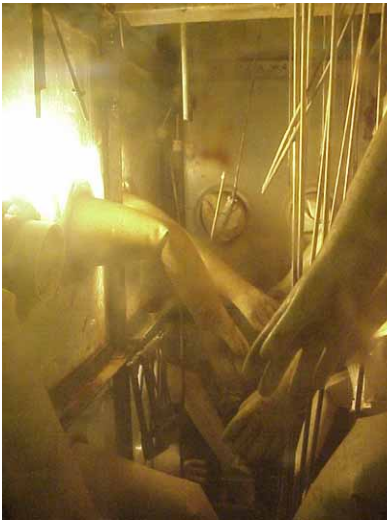
Figure 3 – Many of the chemical systems are located in large gloveboxes within the process facility. Glovebox HC-7C (above) once contained many large Plutonium product storage tanks that have now been removed by the project.
