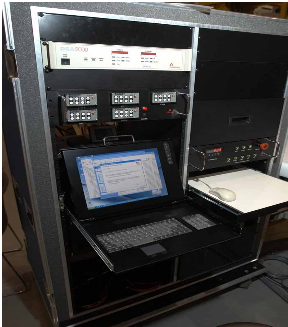
Figure 7 – Operating console and electronics equipment rack
