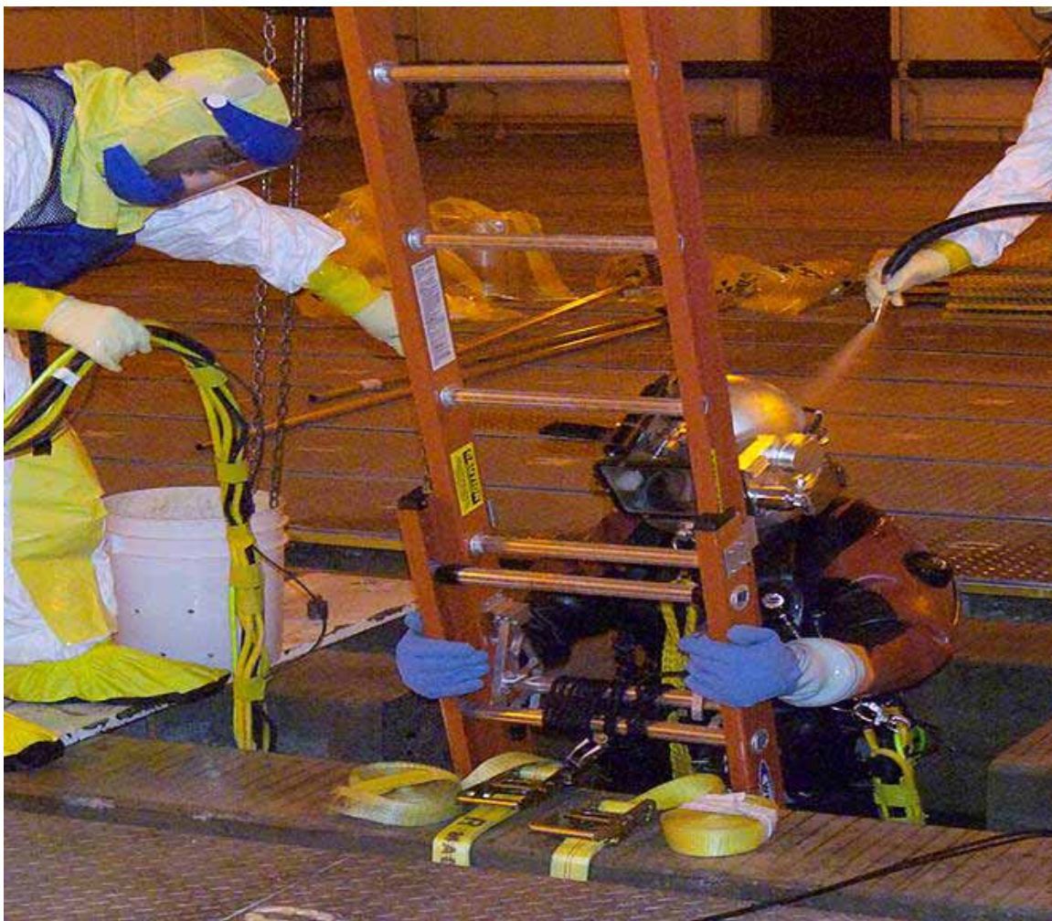
Fig. 3. Diver entering basin through a diver access point
