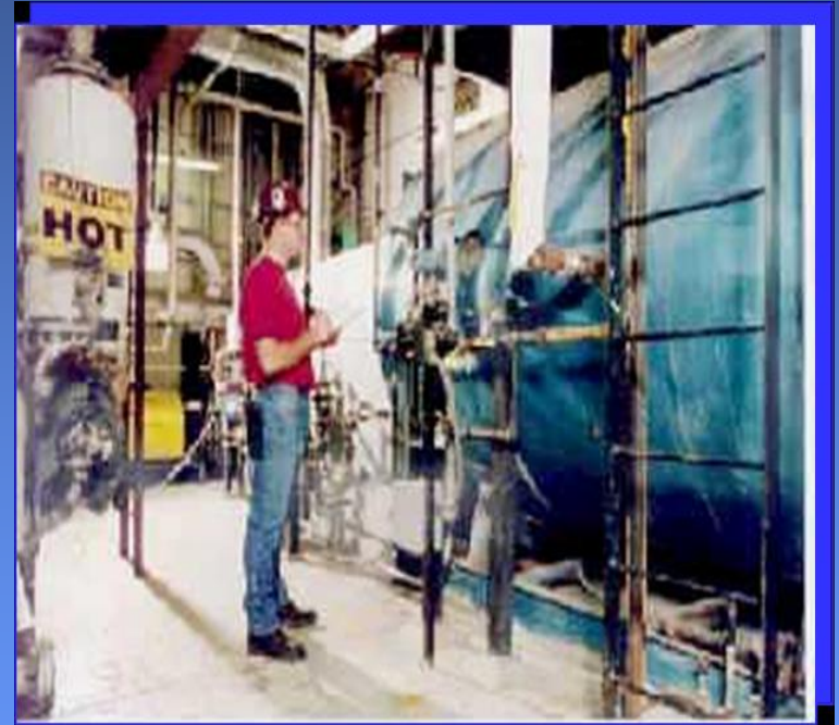
Boiler at DSSI
