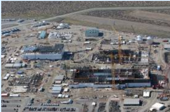
Hanford Waste Treatment Plant Washington State.
