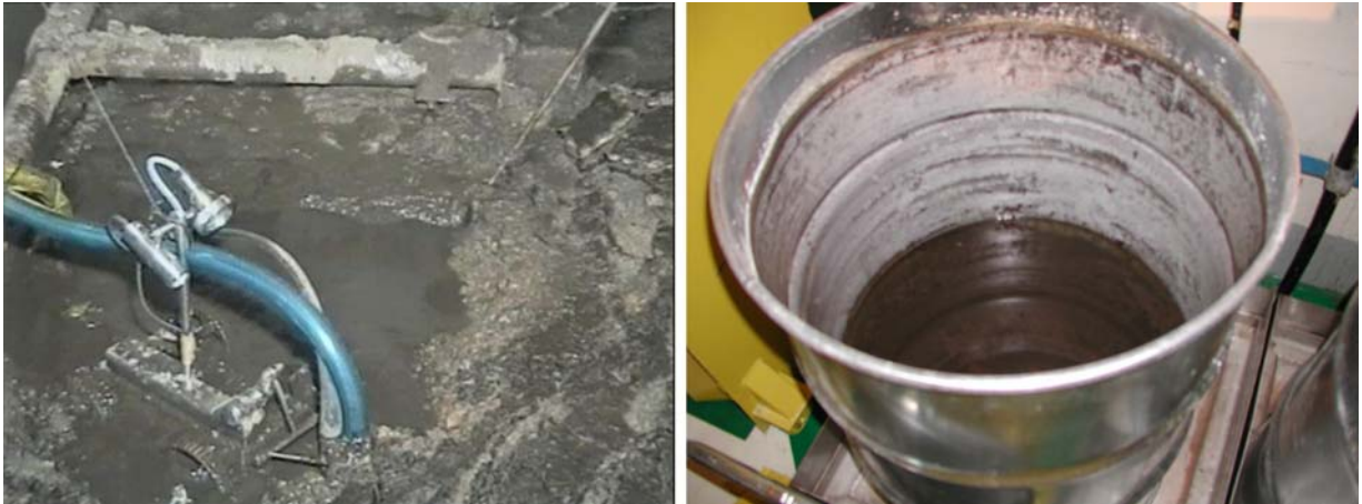
Fig. 3. Removal of the sludge from the "TR" tank by a remote operated vehicle and the sludge collected in the drum
