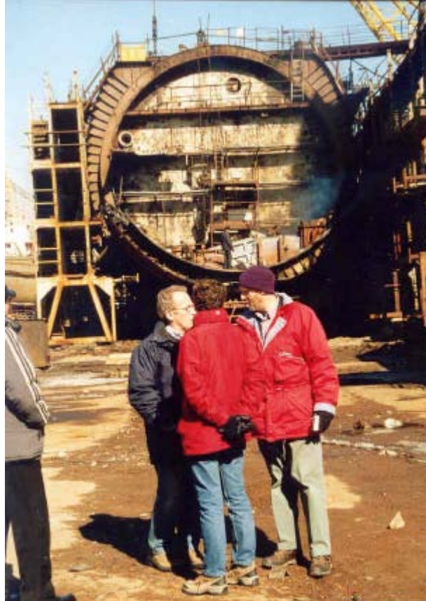
Fig. 3. An Oscar-I Class submarine with the forward block completely removed and the forward bulkhead of the 3-compartment unit being prepared
