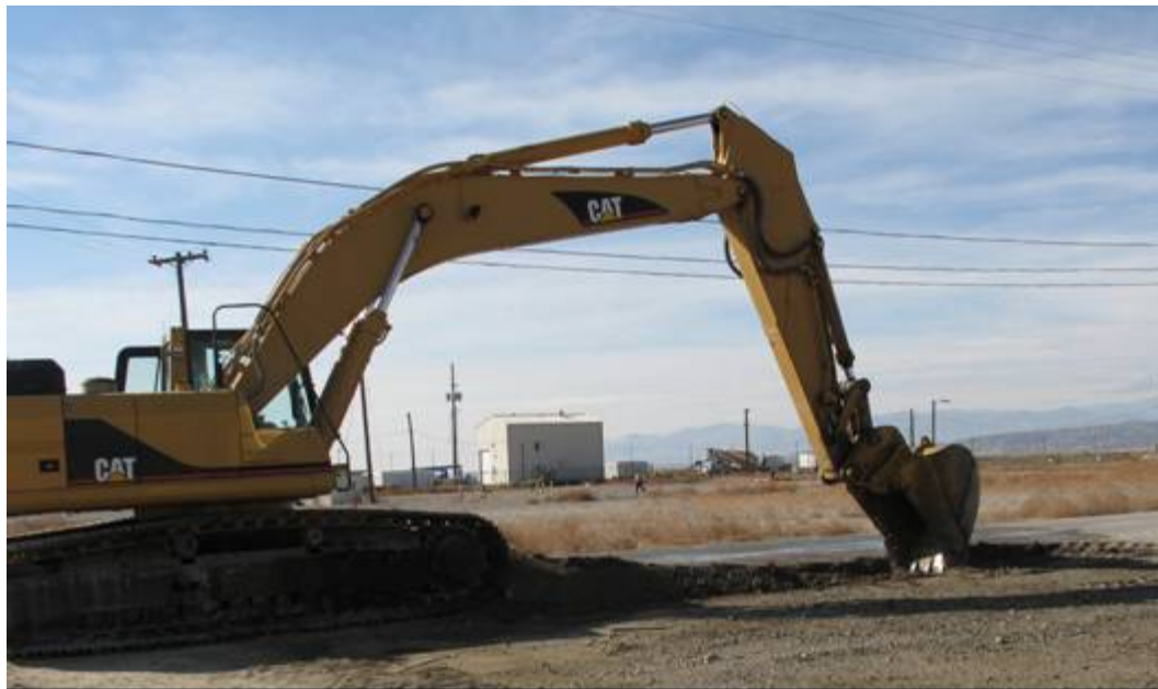
Fig. 5. Real-time remediation process showing the pre-excitation survey, marking of the excavation boundary, removal of contaminated soil
