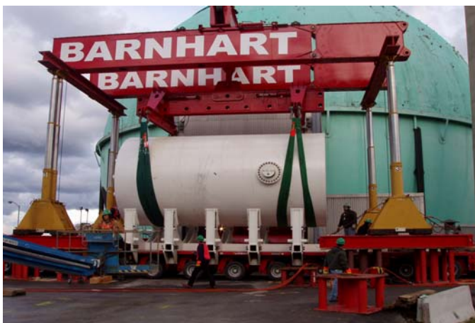
Fig. 4. BRP reactor package loaded onto a heavy haul trailer using hydraulic jacks
