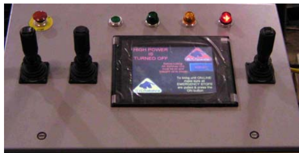
Fig. 4. Typical control panel
