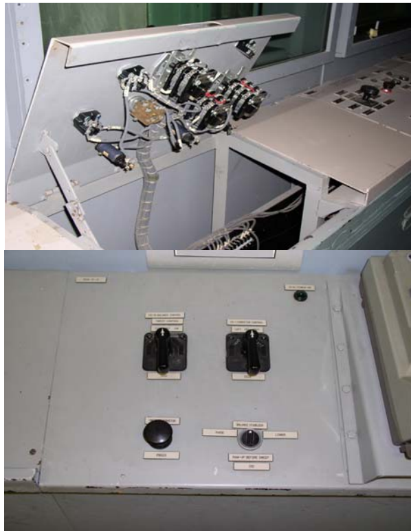
Fig. 3. Underside and top of control panel
