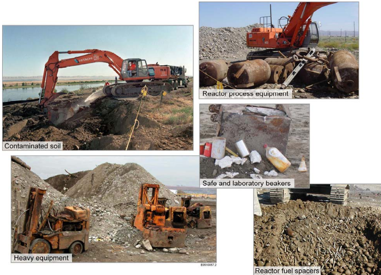
Fig. 3. Excavation of contaminated material from waste sites and burial grounds near the Columbia River
