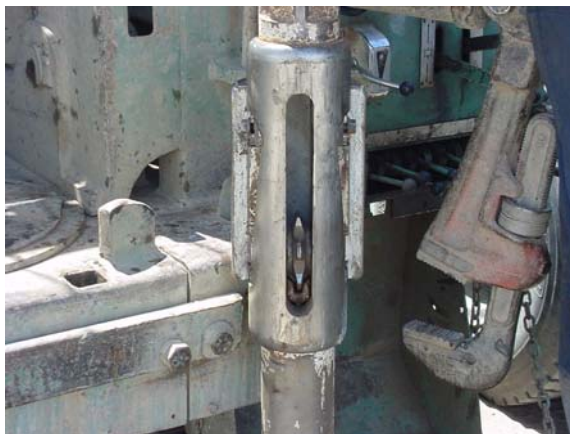
Fig. 3. A mechanical perforator is ready for use in an older Hanford single-cased well.
