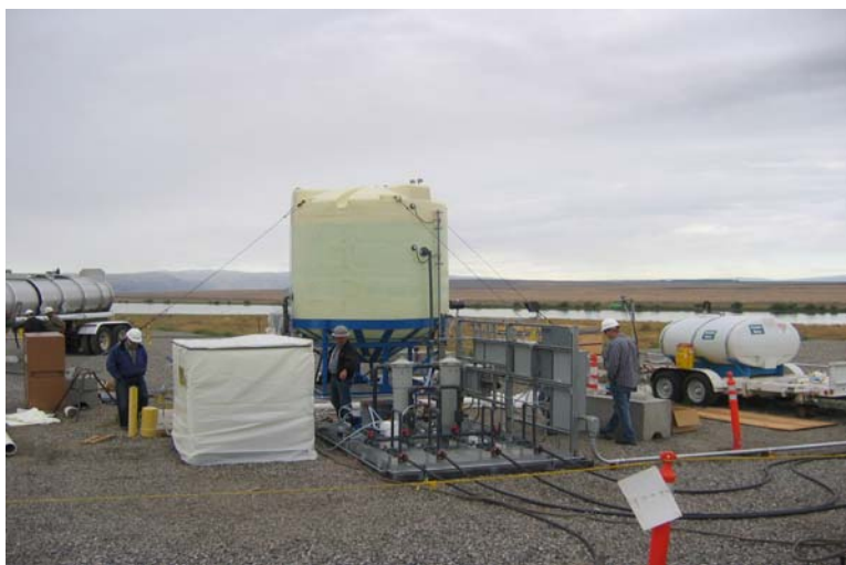
Figure 2. Treatability test equipment, including an above-ground Mixing tank, has been installed in the 100 K Area.
