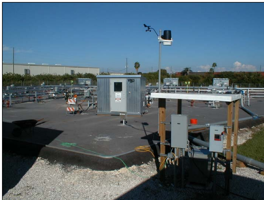
Fig. 1. Area A ET-DSP power delivery system and well field
