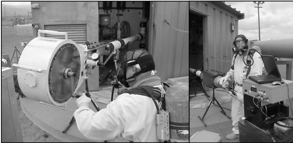
Fig. 3. Photo of the final Pipe Explorer™ equipment configuration used. The pane on the left shows the membrane canister, while the right pane shows the PNG winch and cabling configured with the Pipe Explorer™ canister extension.
