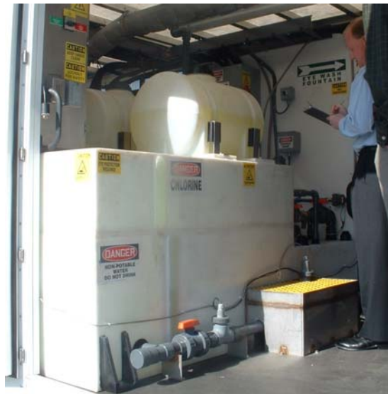
Fig. 8. The on-board disinfectant chemical solution supply system tanks and other components
