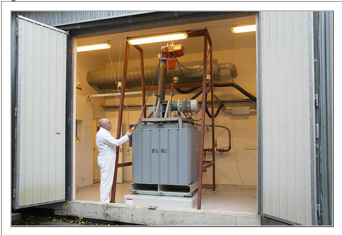
Fig. 2. Waste container with filling and agitator equipment
