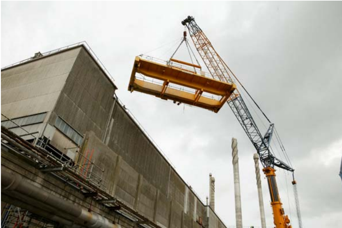
Fig. 4. 50-ton lift – the chassis of the redundant crane was the heaviest lift and took seven hours to safely balance before lifting
