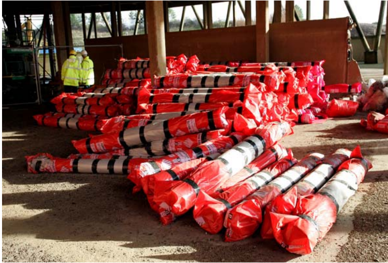
Fig. 2. Asbestos pipe from tower 1 to be containerized
