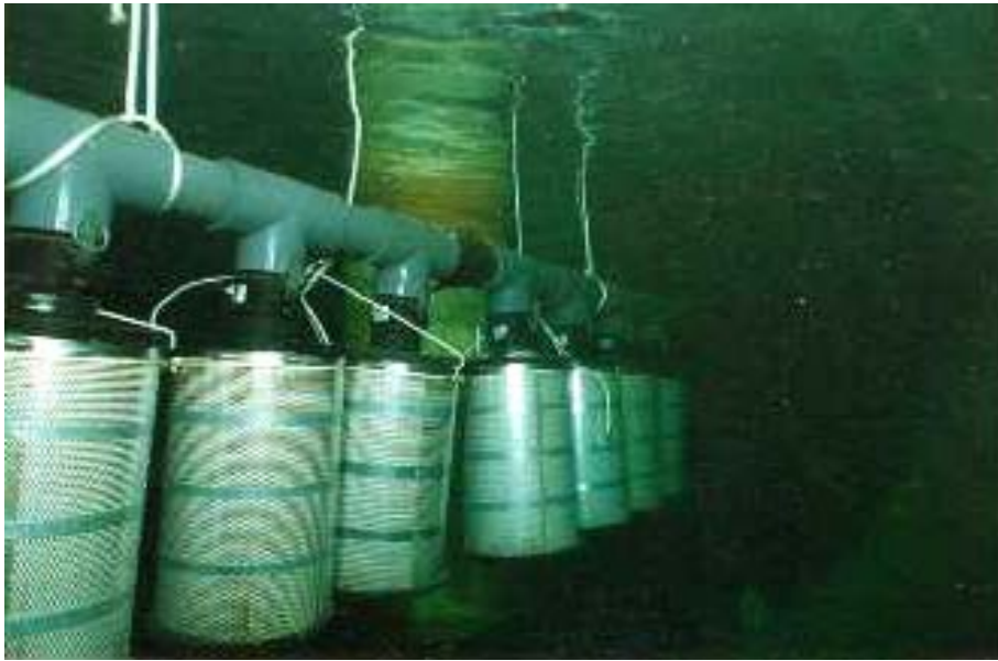
Fig. 3. UCC vacuuming filtration system underwater manifold
