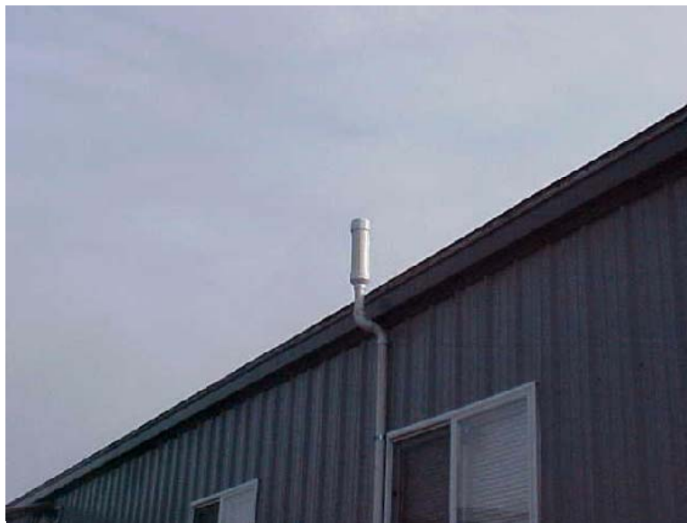
Fig. 8. Lightning detection antenna of the StormTracker system
