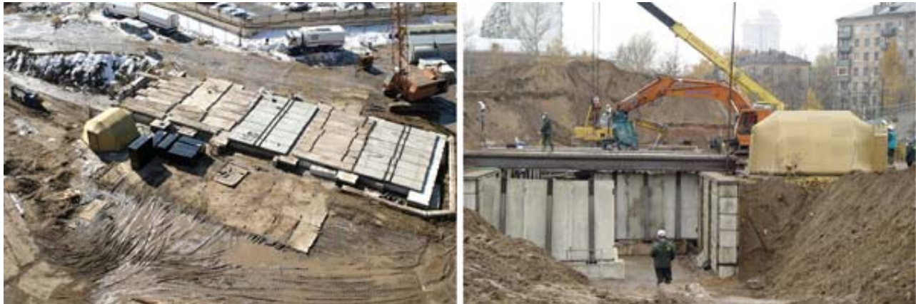
Fig. 2. Shielding structure: top view (a) and view from the labyrinth (b)
