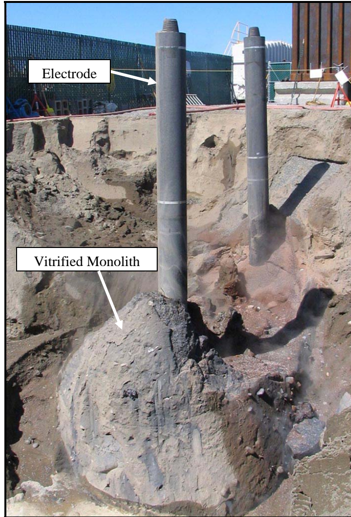
Fig. 5. Vitrified monolith after partial excavation to promote cooling and sampling. Two graphite electrodes are visible extending upward from the monolith.
