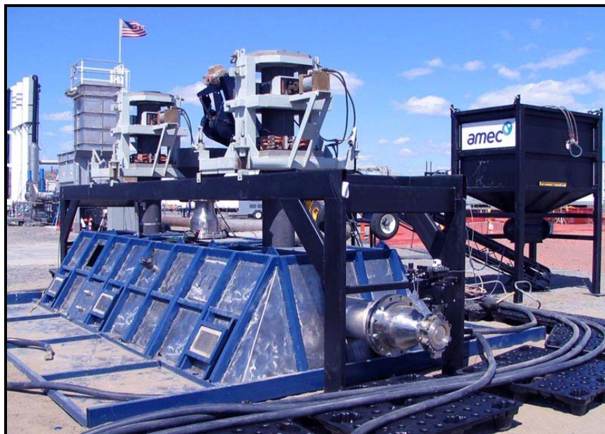
Fig. 3. GeoMelt® SPV™ off-gas containment hood, electrode feed assembly and overburden delivery system.
