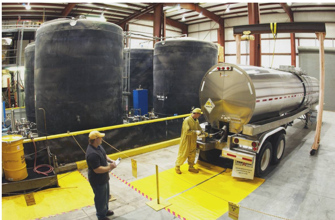
Fig. 1. Tanker receipt bay with four, 10,000 gallon nominal capacity storage tanks.
