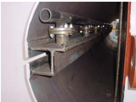
Fig. 3 Interlock injection manifold
