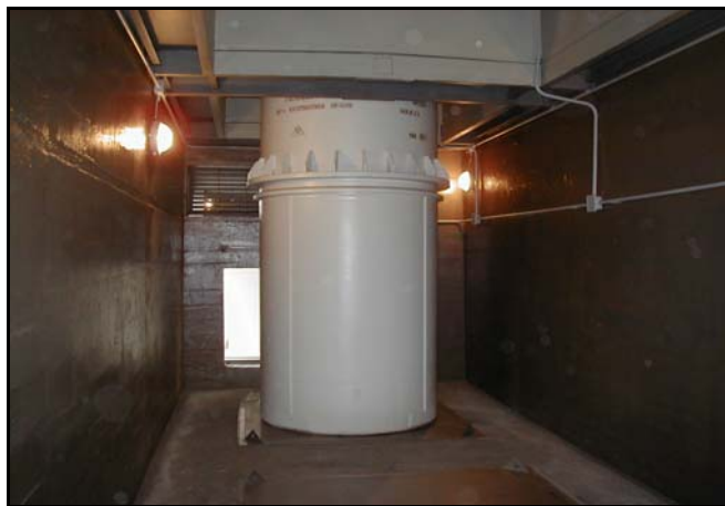
Fig. 2 TUK-108 Prototype Cask in one of the 19 storage cells during cold-testing of the Transshipment/Interim Storage Facility, June 2003.
