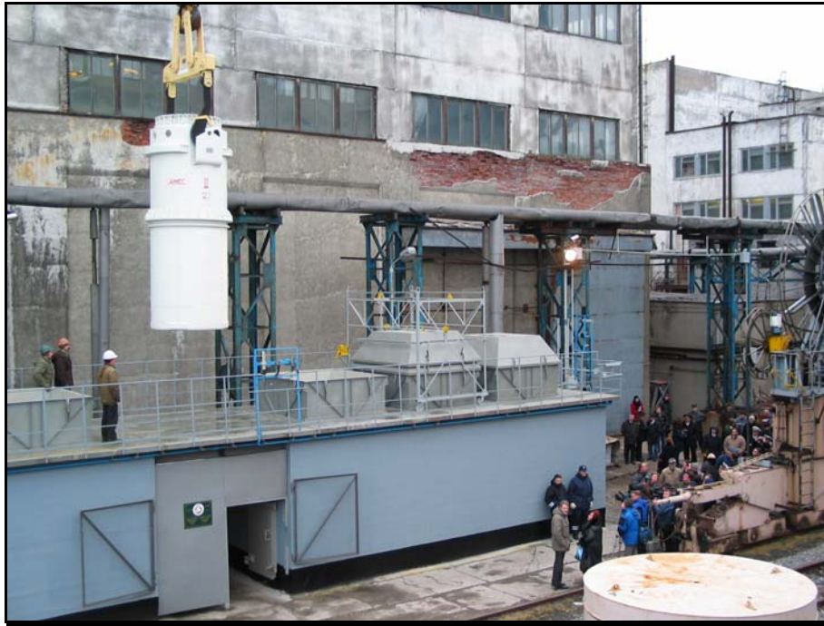
Fig. 4 TUK-108 Prototype Cask being placed in the Storage Facility during the November 2003 Project "Promotional Event" noting the completion of the Facility construction.
