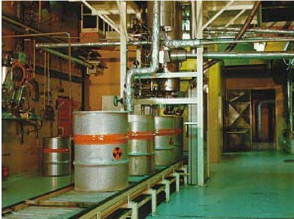
Fig. 1 VUJE bitumenation plant
