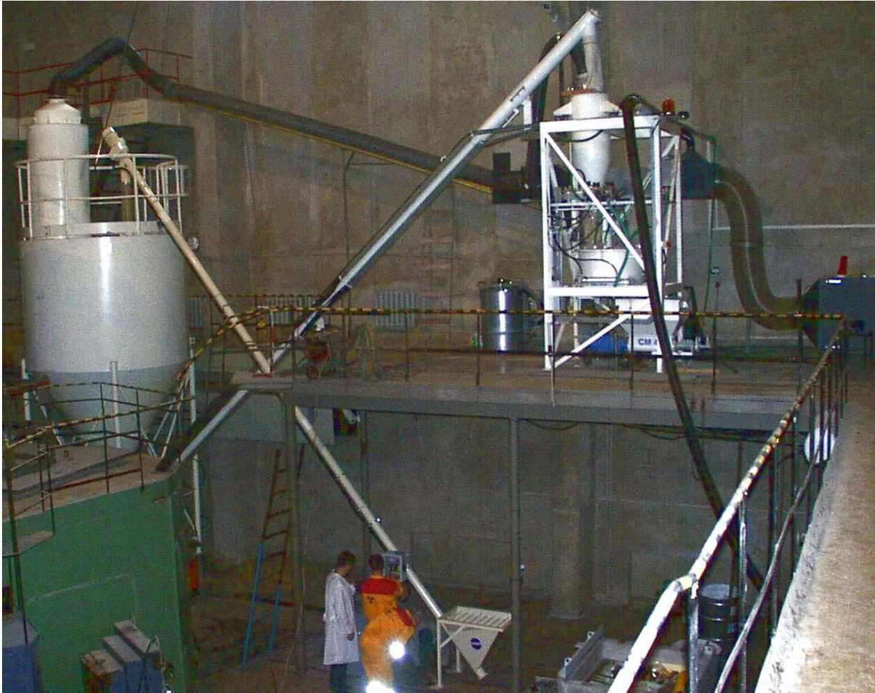
Fig. 2 The cementation facility for immobilization of tritiated water, Salaspils, Latvia.
