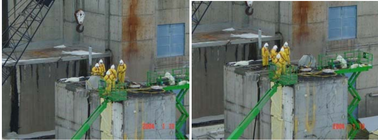
Fig. 4 Images during segmentation – left photo depicts shrouded concrete saw at the beginning of a horizontal roof cut; right photo depicts the shrouded wall saw at the end of a horizontal roof cut. ( Notice saw receiver -- designed to capture slurry released by the exposed saw blade as it begins or completes the cut. )
