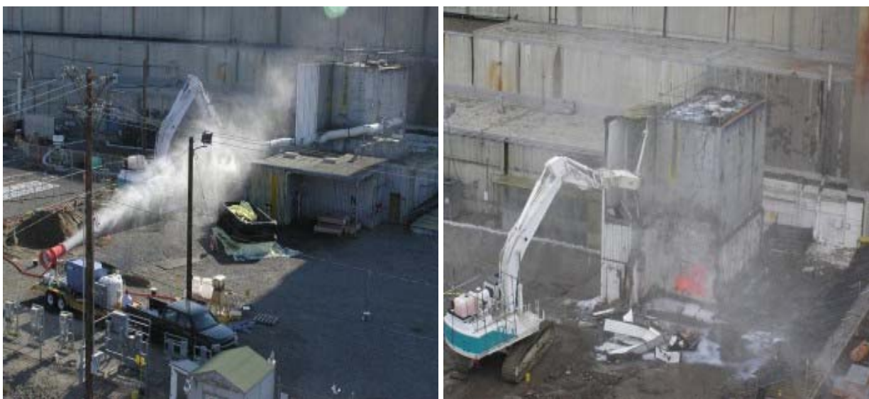
Fig. 3 Images during demolition – left photo depicts demolition of the 233-SA Building (note the FOG CANNON ™ in lower left of the image and the ERDF waste container in center); right photo depicts subsequent demolition of the 233-S process hood stairwell.
