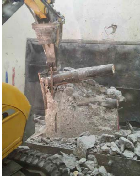
Fig. 3 Crushing of concrete bars and separation of different material by means of a chisel excavator
