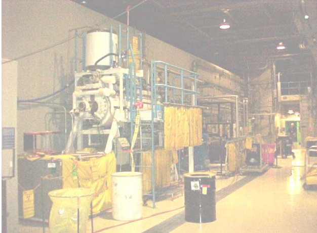
RVR Installed at Callaway
