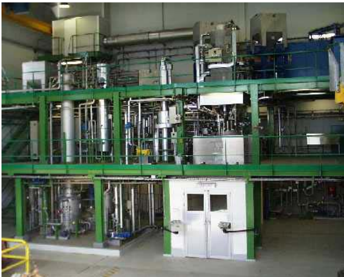
Fig. 1 General view of the Vitrification facility
