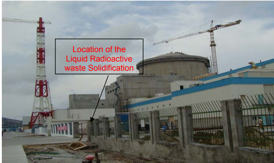
Fig. 3 Tianwan Reactor Unit 1 incl. machine room in the front and the waste treatment area left to the reactor
