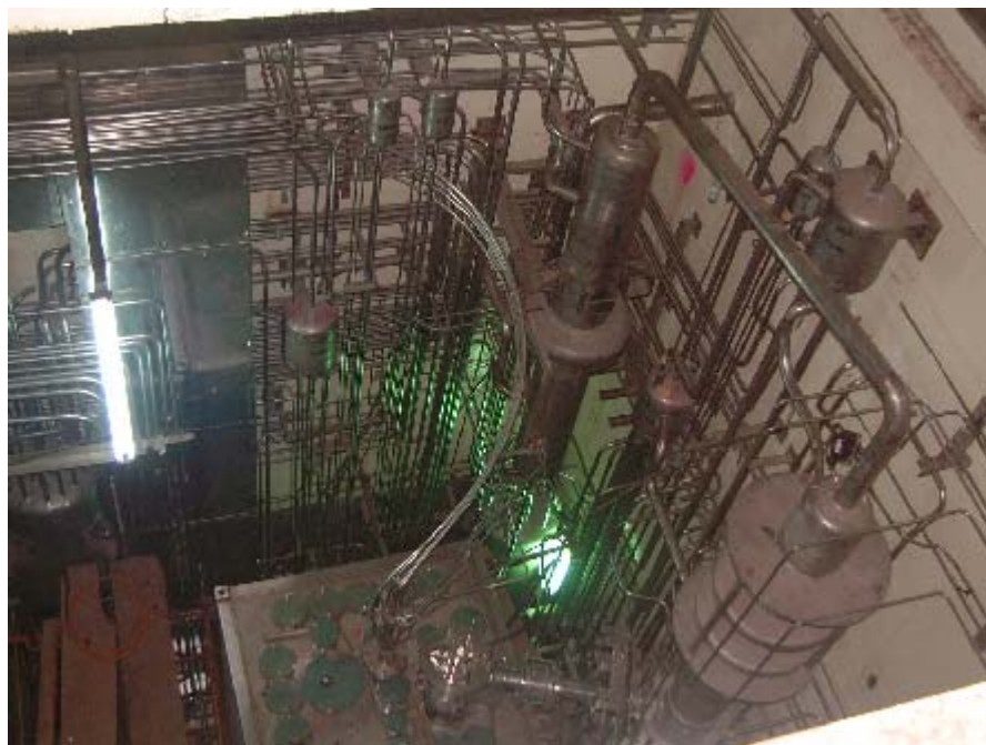
Fig. 4 A typical view of pipe routing and equipment layout on the top of JHCM
