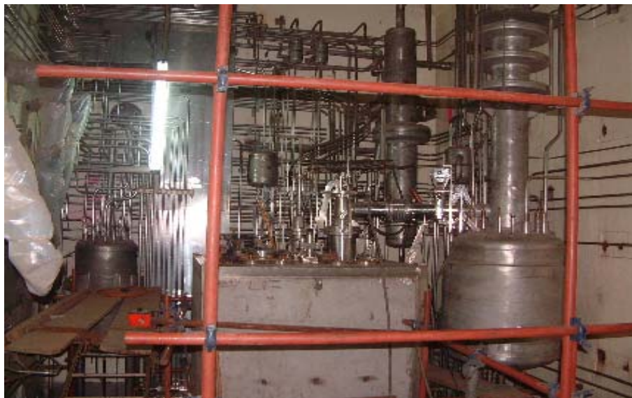
Fig. 3 Top View Of JHCM & Associated Equipment housed in the Melter Cell
