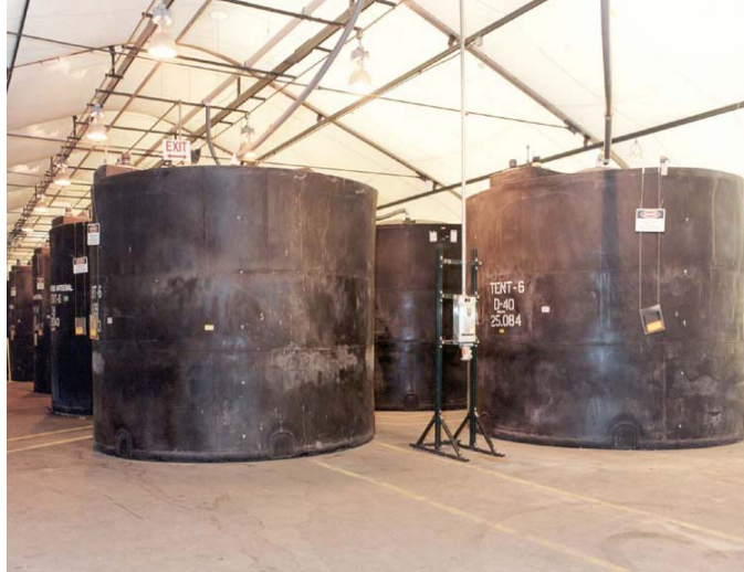
Fig. 3 10,000 gallon tanks used for sludge storage
