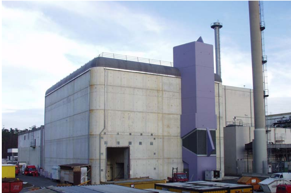
Fig. 1 VEK construction site (December 2003). front view of process building with characteristic structure of canister storage cooling air channel
